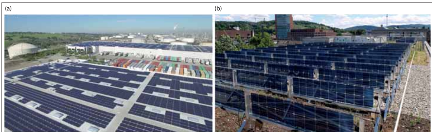
Figure 4. (a) 10 MWp bifacial fixed tilt installation by sunpreme (USA) [42] and (b) bifacial vertical installation by Solarspar (Switzerland) [43]
