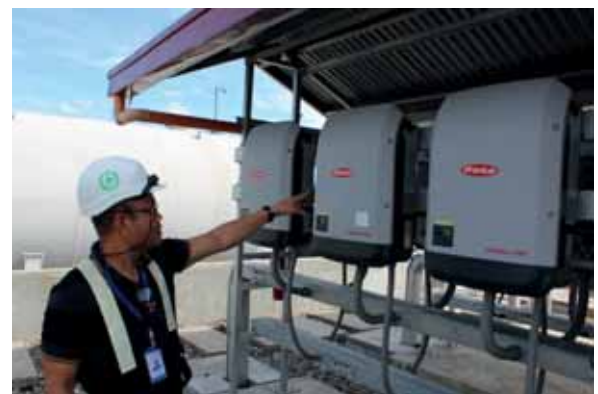
The project uses 60 Fronius inverters
